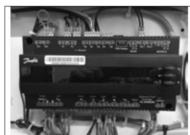
Picture 4 : Normal wiring
