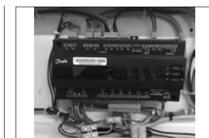
Picture 5 : Temporary wiring
